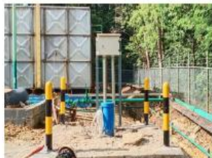
Instalasi Positive Junction Box
