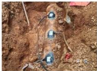
Bonding kabel negative
