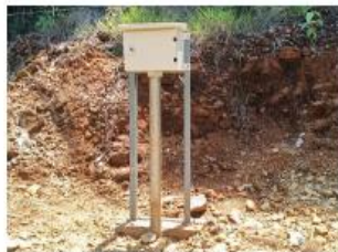
Instalasi Negative Junction Box
