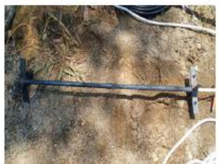
Instalasi Anode Centralizer
